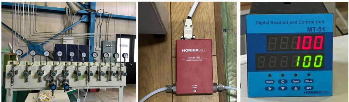
Figure 7. Gas supply station and mass flow controller.
